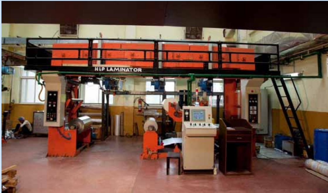
Laminator - Conversion Plant
